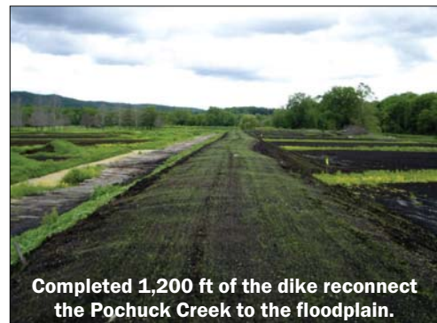
100 ft section of this dike gave way to flood waters destroying croplands in Orange Co.
