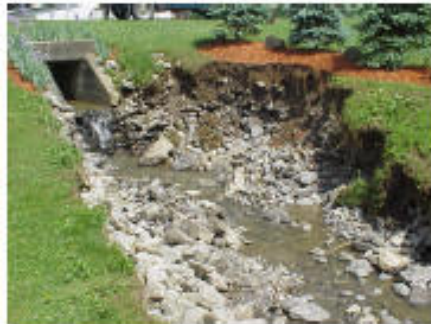
Town of Sheldon Storm Damage
