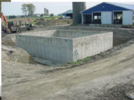
Methane Digesters NYSERDA Grant to the Town of Perry.
